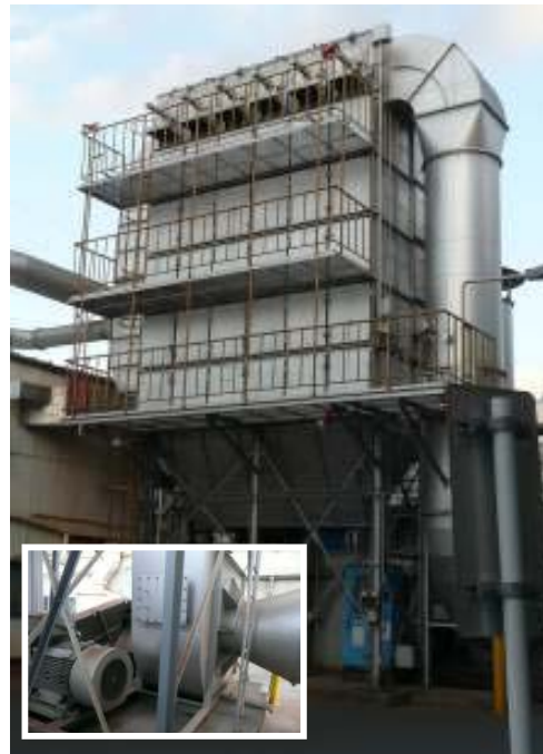
Foundry dust collector
