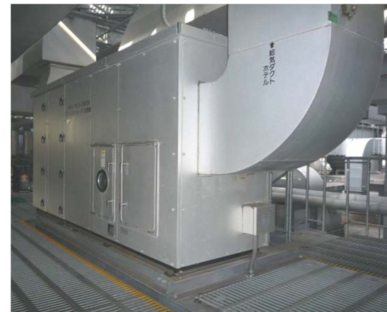
Air handling unit (AHU)
