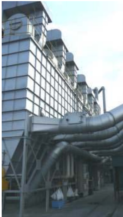
Dust collector of wood processing
